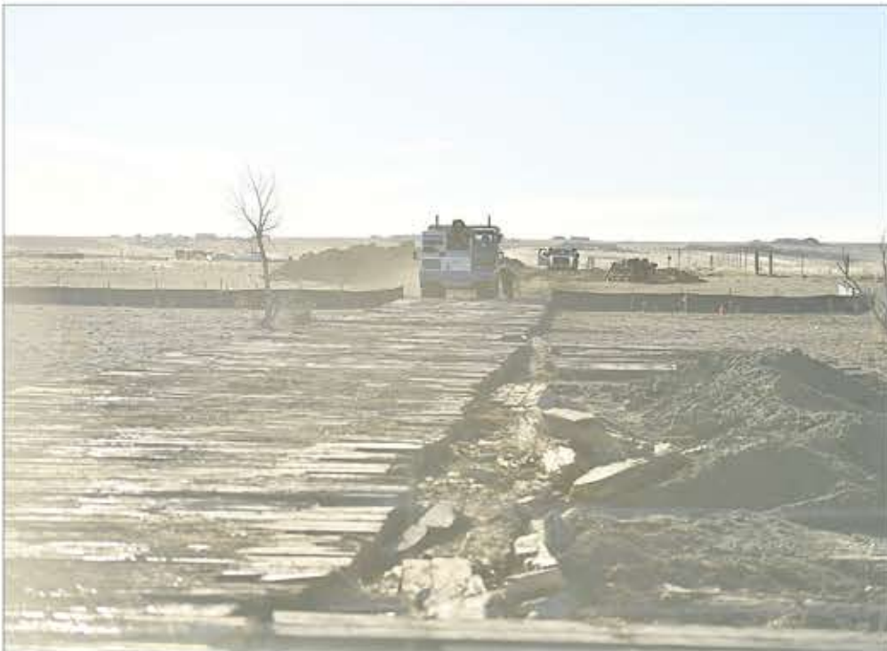
The Magellan Pipeline expansion for petroleum product distribution to Denver International Airport, including jet fuel, is being placed within 30- to 50-foot-wide right-of-way easements.
